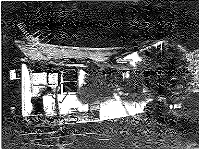
Above: When wiring goes bad. A house gutted by fire at Brukungu.
